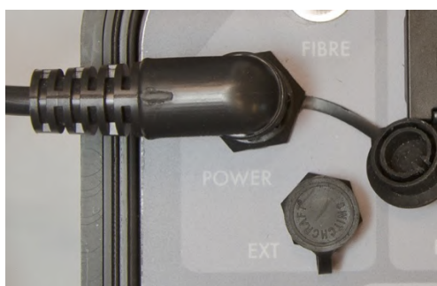
Control Station power cable plugged in and secured with plastic collar
